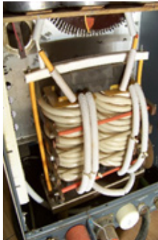
Fig. 11. A part of HV rectifier with cooler platelets
